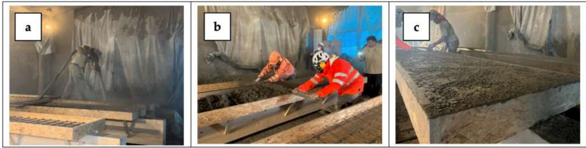
153 154 Fig. 3. Example of a Shot-Earth and timber coupling: (a) Shot-Earth projection in wooden formwork to 155 realize 9 m length beams, (b) surface flattening, and (c) Shot-Earth consolidation
