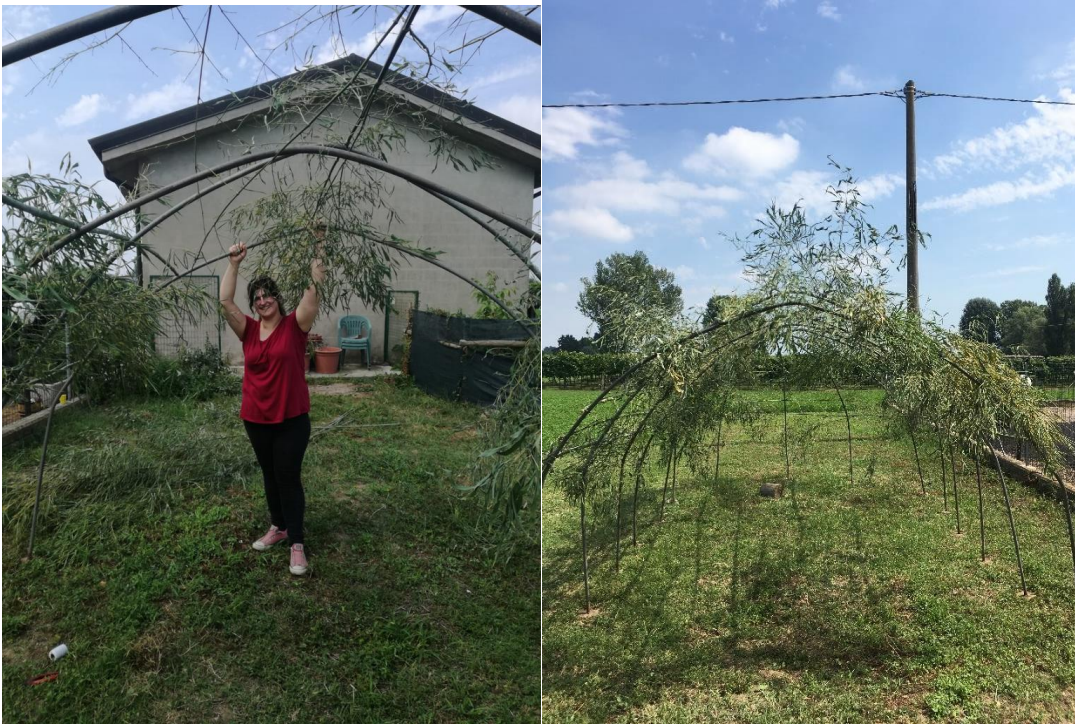
Figure 7a: bamboo drums installation on the metallic structure. Figure 7b: particular of bamboo cover with leaves on.
