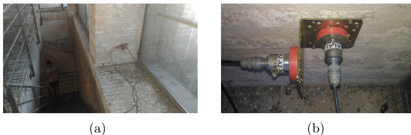
Figure 3.21: Fortress: typical installation of piezoelectric accelerometers.
