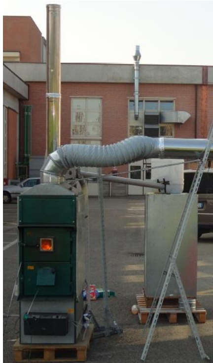
Figure 3. Pellet combustion facility
