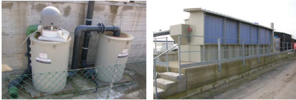
Figure 17-40: Drum and Scrubber
