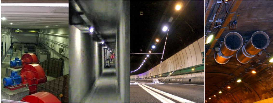
Figure 2.2: Details of the Mont Blanc tunnel ventilation system: (left to right) interior of the ventilation station on the Italian side; underground fresh air channel; fresh air supply vents along the sidewalk; a pair of jet fans.
