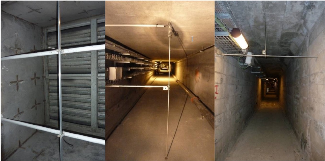
Figure 2.3: Detail of the installation of sensors in the ventilation channels.
