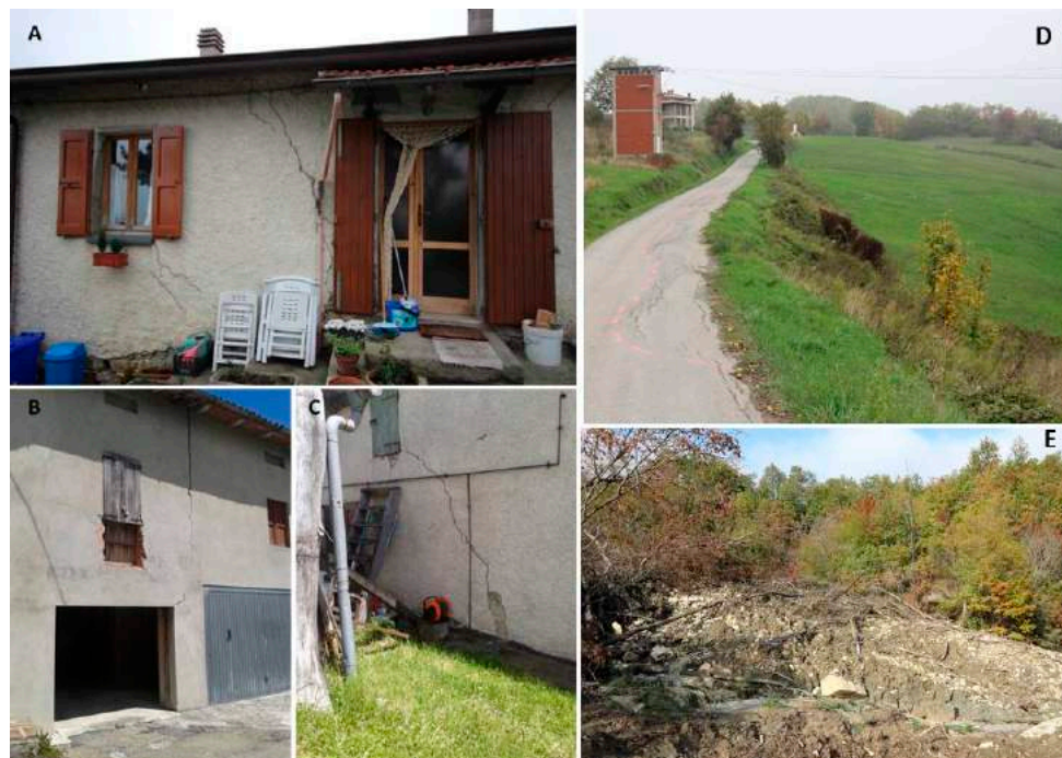
Figure 12. Evidence of movement on Pianestolla buildings (A–C) and in correspondence of the sectors \delta (D) and \epsilon (E).
