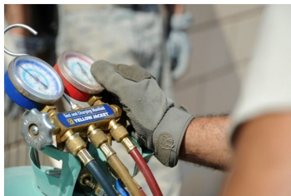
Figure 3 A technician controlling a Ventilation System
