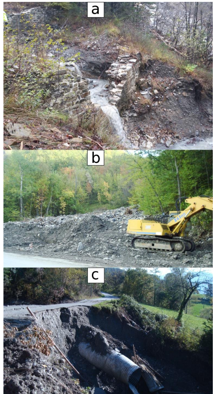
Fig. 5 – Example of effects on infrastructures in Parma province: a) check-dams cut-through by debris flows; b) road overrun by debris; c) erosion and cut-through of the road track.
