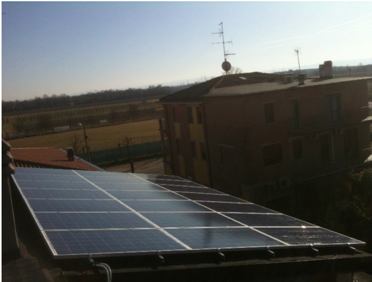
Figure 1. PV power plant.
