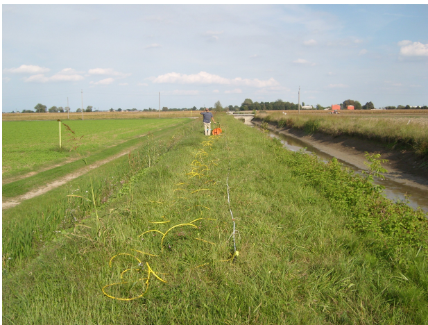
Figure 1: Earth levee and water channel (on the right) in test site A at the end of the irrigation season.
