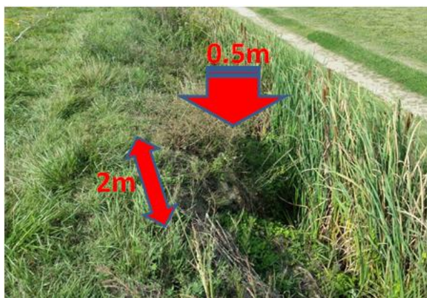
Figure 3: Small levee subsidence observed in test site A.
