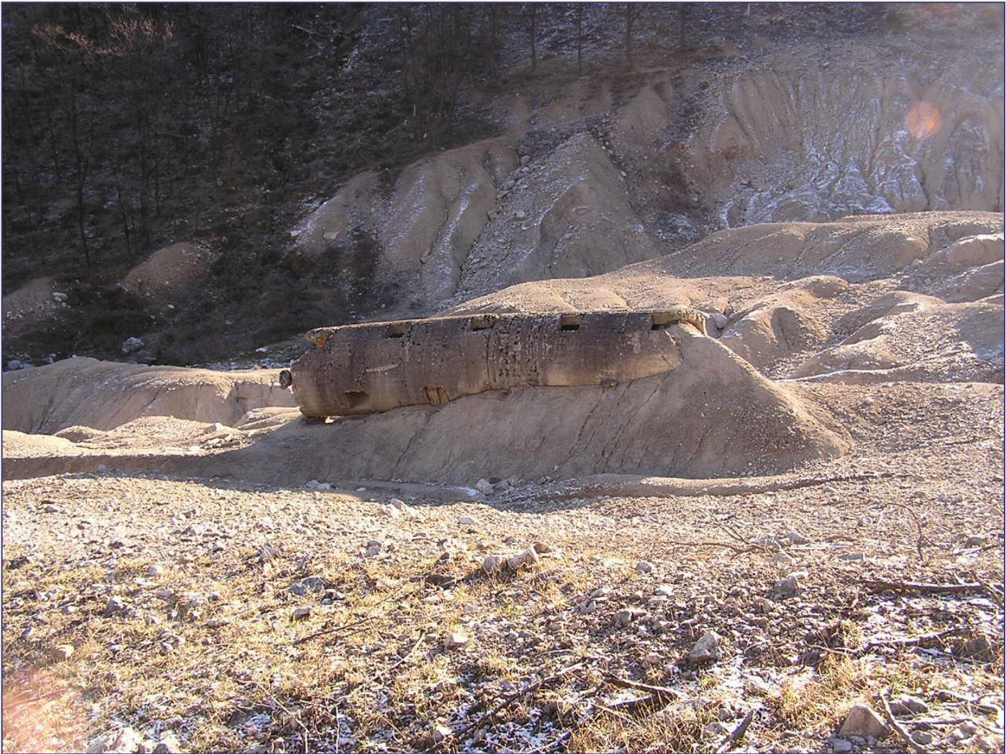
The remains of the Sgorigrad tailings dam with a fallen overflow tower.
