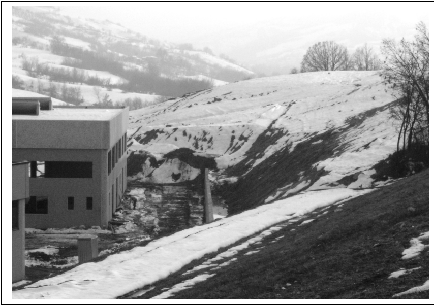
Fig. 5 – Slope cut at the foot of the Ca' Bonettini landslide and containment wall (March 2004)
