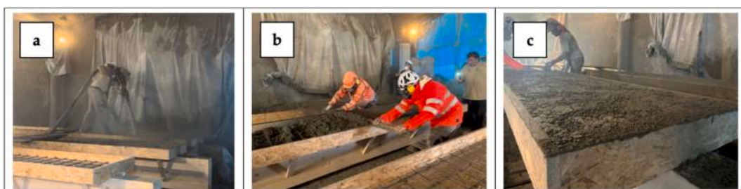
Fig. 3. Example of a Shot-Earth and timber coupling: (a) Shot-Earth projection in wooden formwork to realize 9 m length beams, (b) surface flattening, and (c) Shot-Earth consolidation.
