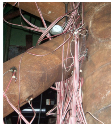
(c) Bulge at the end of the compression brace of specimen CFST-6s
