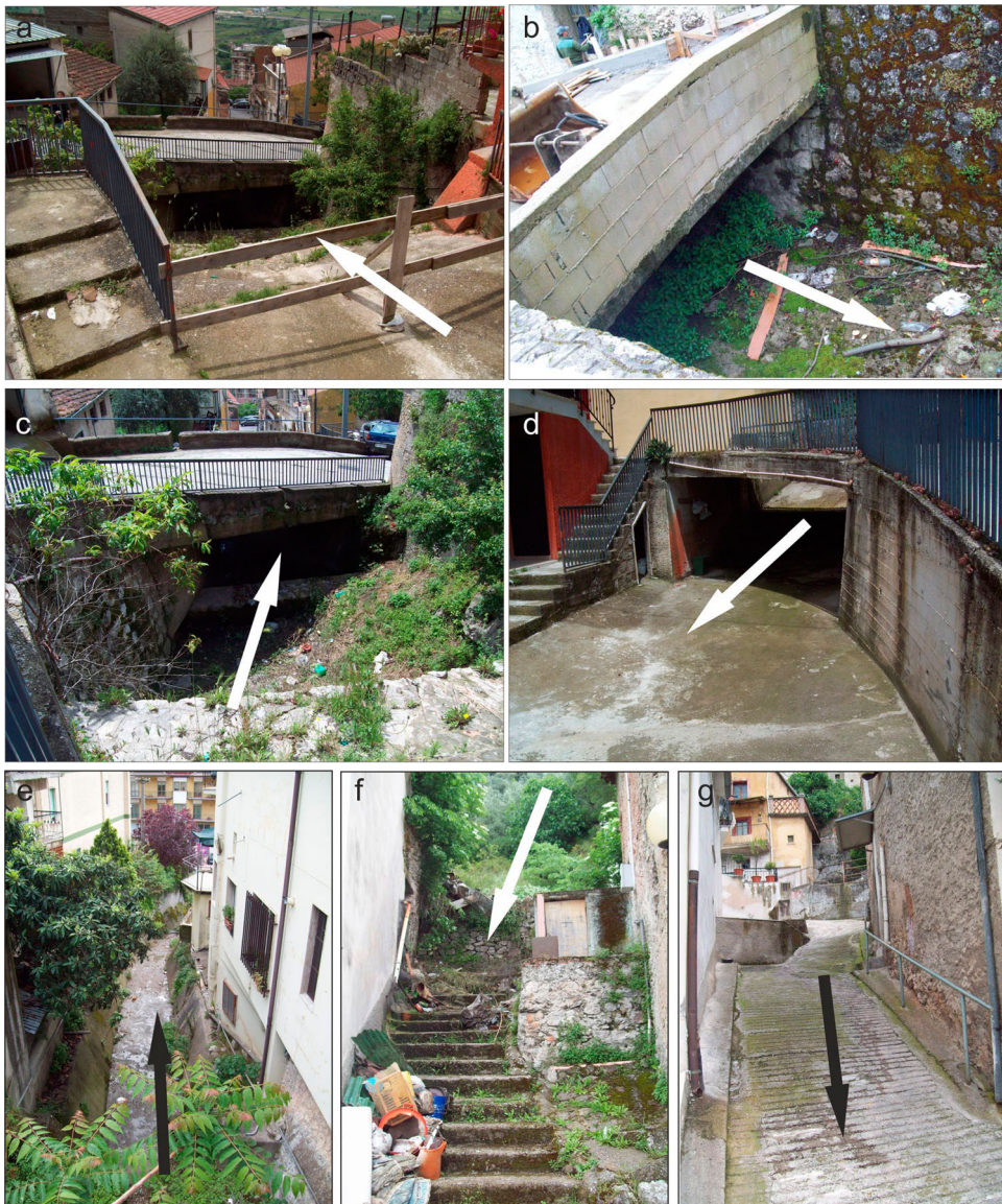
Figure 4. Examples of hydraulic critical points in Sala Consilina: (a), (b) (c) and (g) the main stream is channeled underground; (d) and (f) the stream re-emerges, but its bed has become a road; (e) the stream has a very small cross-section and is completely surrounded by houses.
