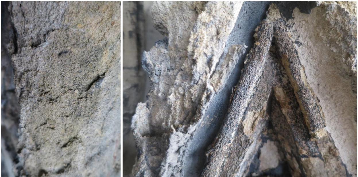
Figure S10. Intermediate restoration state, during the cleaning procedure and before treatment application. The rain exposed surfaces marked in red (top figure) have been used for consolidation purposes in the frame of this work. Bottom figures exhibit the differences in densities and decay patterns.
