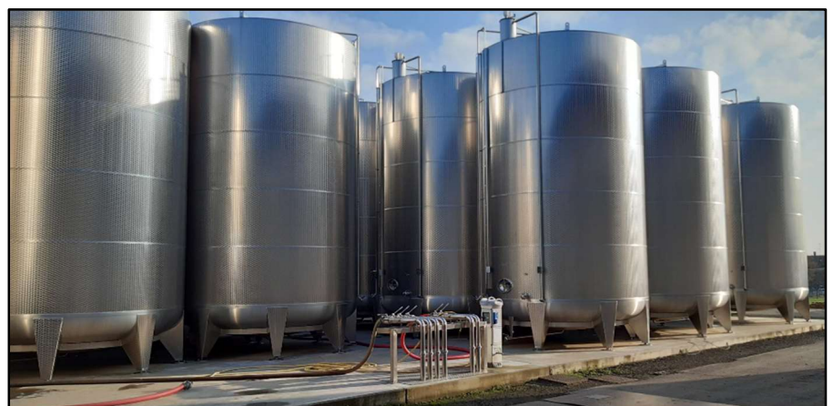
Figure 10: Raw materials external storage steel tanks (Scandiano site)
