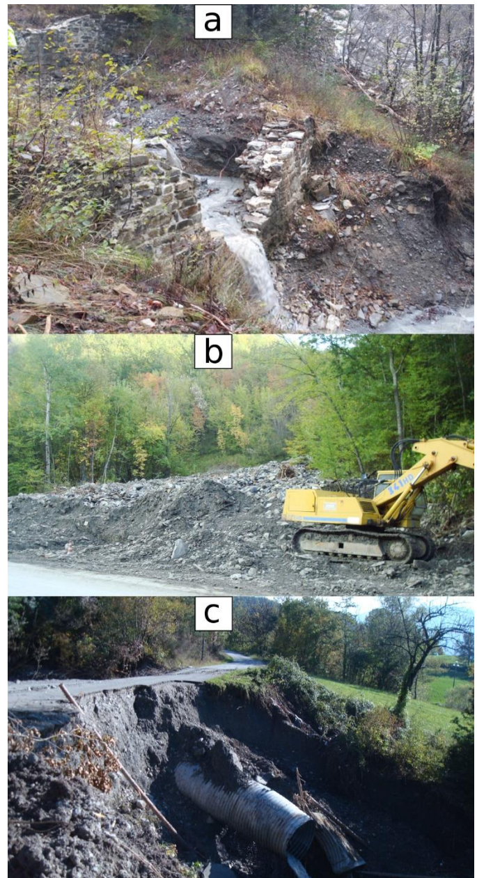
Fig. 5 – Example of effects on infrastructures in Parma province: a) check-dams cut-through by debris flows; b) road overrun by debris; c) erosion and cut-through of the road track.
