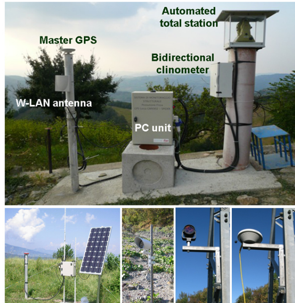
Fig. 2. Integrated monitoring system for unstable slopes: master unit at the top; below GNSS benchmark for continuous monitoring, monitoring reflector and reference prism/GNSS respectively
