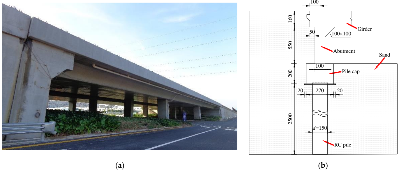
Figure 2. Engineering background: (a) overall view of the IAB; (b) details on the girder, integral abutment, and pile (unit: cm).
