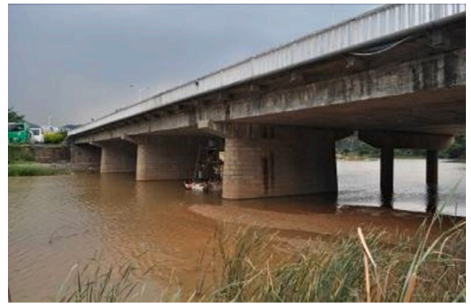
Fig. 3. View of Zhangzhou Shili Bridge. Source: Photo taken by the author Junqing Xue.
